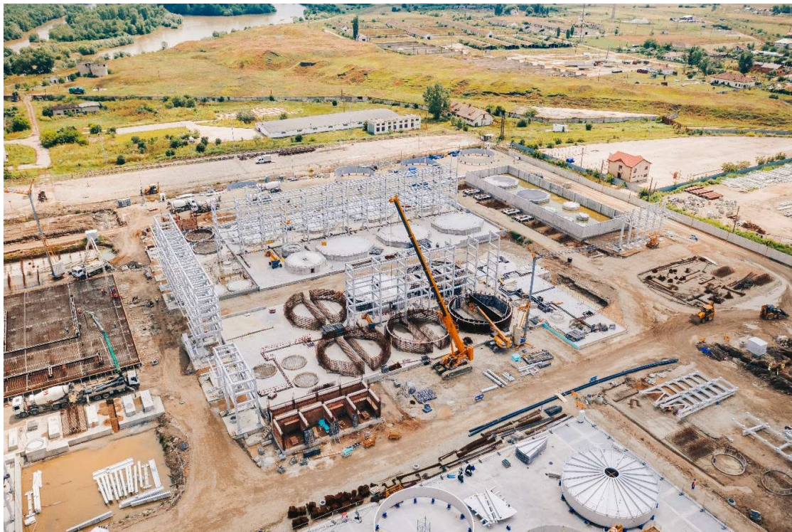
PICTURE CAPTION: CURRENT AERIAL VIEW OF THE CLARIANT SUNLIQUID CONSTRUCTION SITE IN PODARI, ROMANIA (PHOTO CREDITS: CLARIANT)
